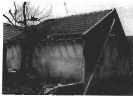
Figure 7. The scratch mark and roof tile damage are used as the estimate of tsunami inundation (Devanaapattinam, 11^{\circ} 44.567' N , 79^{\circ} 47.317' E ).
