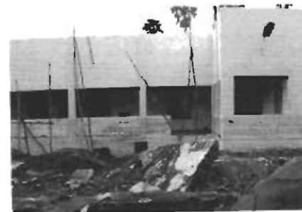
Figure 4. The mud line on the building wall is used as a reliable tsunami inundation level (Pekkalapet, 12^{\circ} 01.708' N , 79^{\circ} 51.950' E ).
